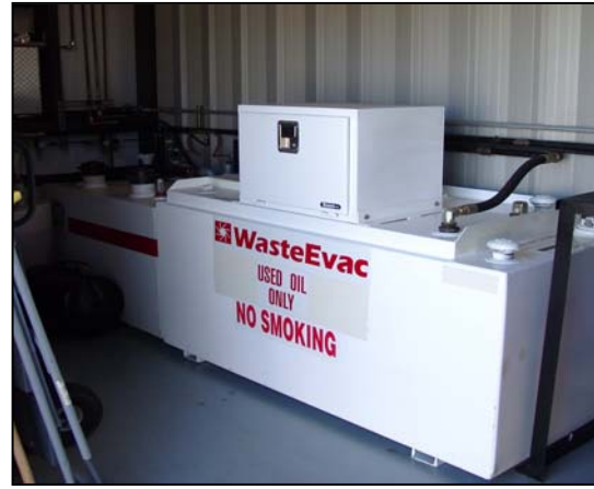
Waste oil storage
