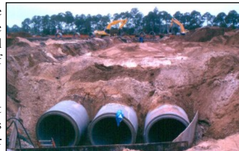
A series of three, 72-inch pipes direct water from Naples Park through TOCGC to wetlands near the river.
