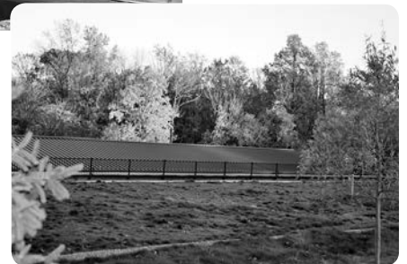
The use of grass on top of the roof necessitates the need for ongoing irrigation at Merion Golf Club. The growing medium was blown in, spread by hand, and then smoothed by machine. Note the waterproof membrane.
